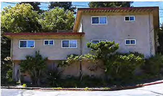
1e. 3-story, 5-unit. WFTS: Hillside cripple wall. Tall crawl space under first floor to accommodate hillside site (note vent openings in wall).
