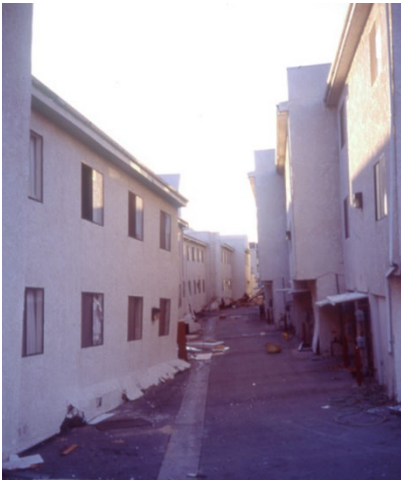
Collapsed and near-collapse 3-story buildings, Los Angeles, 1994 Northridge earthquake (photo: Gary D. Avey)
