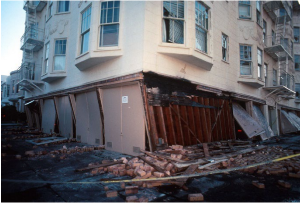
Near-collapse, San Francisco, 1989 Loma Prieta earthquake
