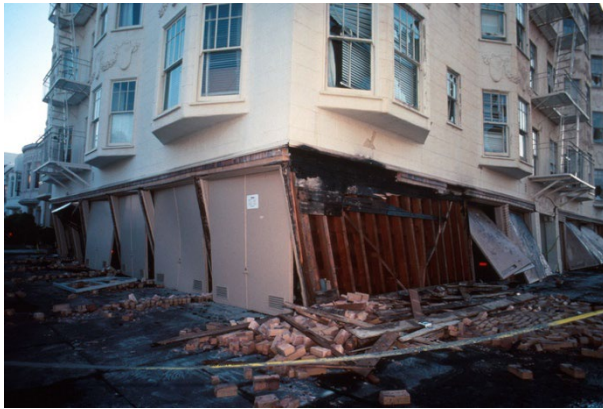
Near-collapse, San Francisco, 1989 Loma Prieta earthquake
